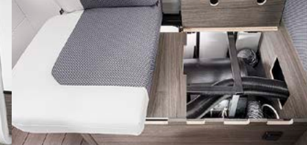
4 Truma diesel heating under the seat bench
