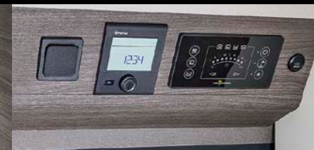
15 Control panel above the sliding door
